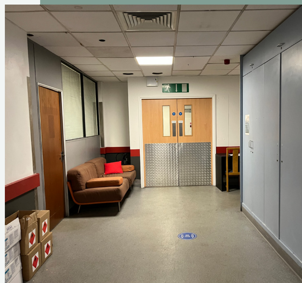
Condition of the floors in back-of-house areas
